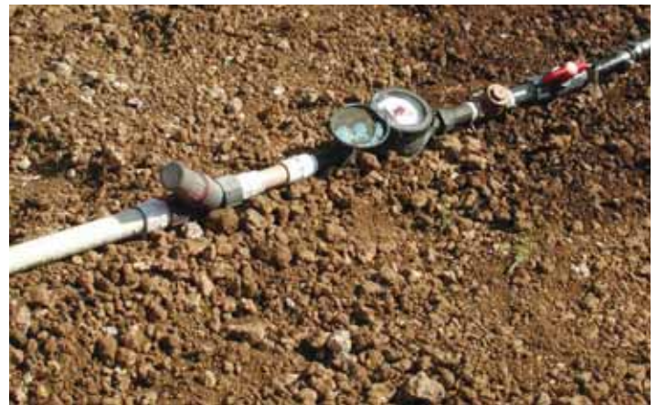
Figure 8. Water meters installed near the field.
