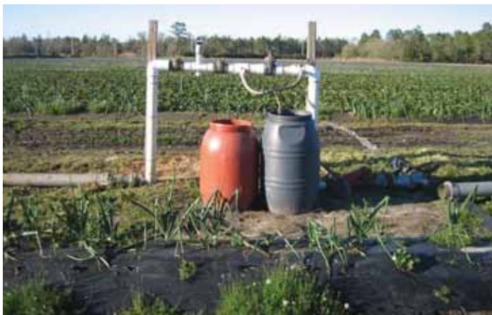
Figure 4. Back-flow prevention made of two ball valves and a vacuum breaker are placed upstream of the Venturi injector. Credits: Eric Simonne.
