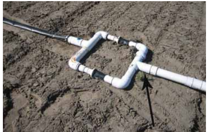
Figure 7. Pressure regulators are installed side-by-side in this system to allow a greater flow rate. Note the small injection port for chemical injection.
