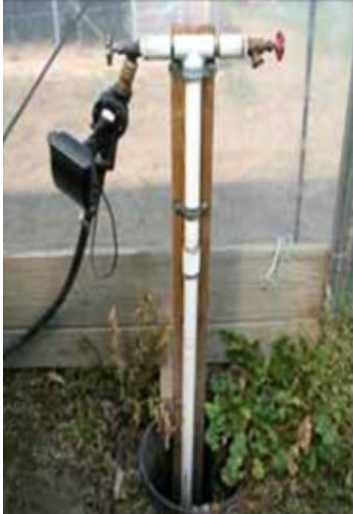
Figure 5: Water supply (vertical standpipe) to the inside of a tunnel showing (left) a faucet used for drip irrigation (with an irrigation timer directly attached to the faucet), and (right) an unused faucet for attaching an irrigation hose (not shown).
