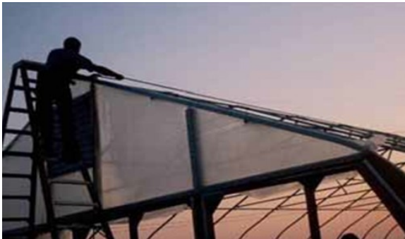
Figure 26: Installing the plastic film to the end wall of a high tunnel.
