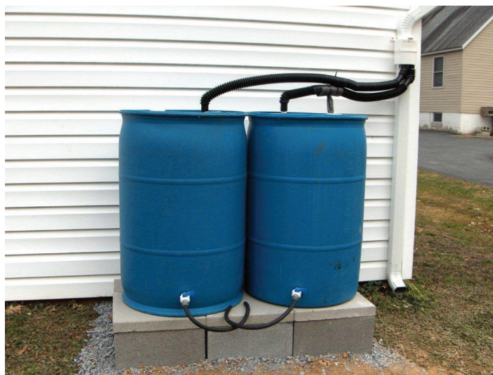
Figure 1. Rain barrel installation collecting from gutters. Credits: Kimberly Moore, UF/IFAS
